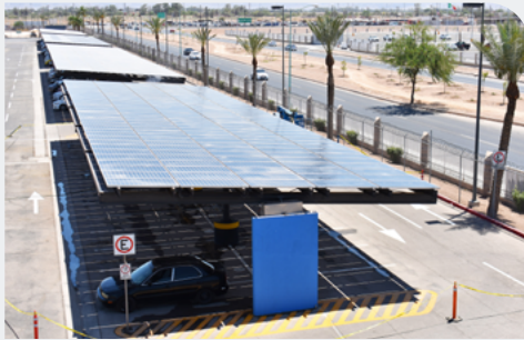
Solar panels installed as part of our 'Carport project' in our Mexicali plant (SPMX1)
