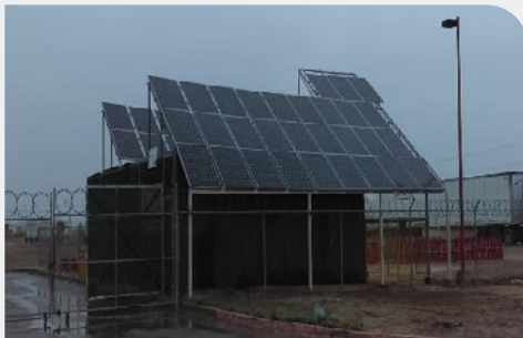
Solar panels installed atop our organic garden
